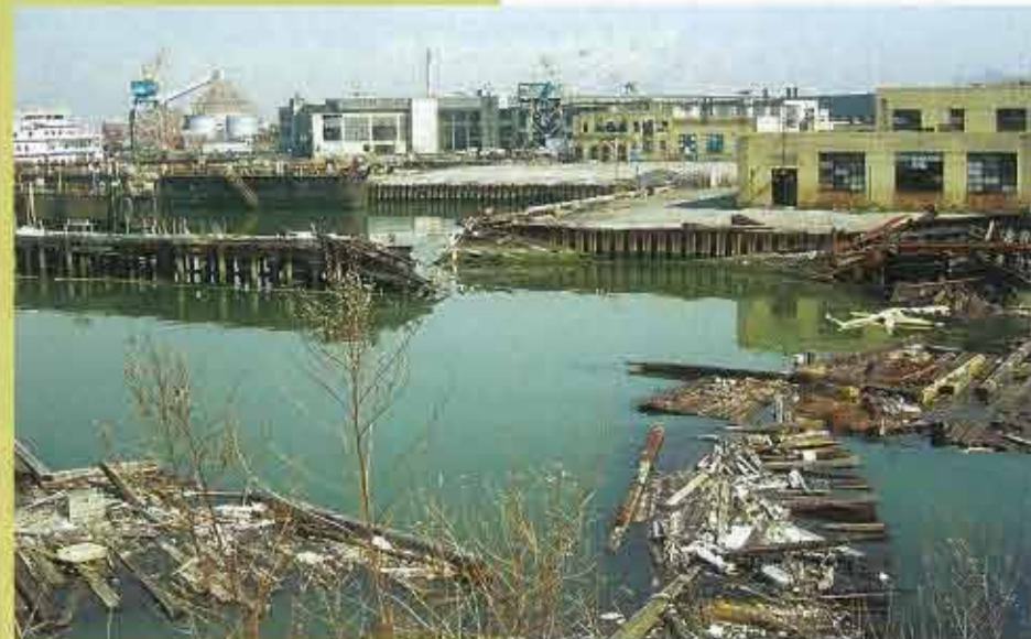
Prior to the park being built, the docks had deteriorated.
